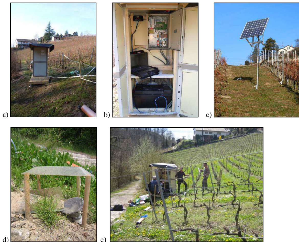
Appendix 1.4: Monitoring station in parcel 2, with a) the house in which are b) a data logger (green device), a power regulator (black device, up left), a GSM modem (grey device, up left in the box) and a battery powered by c) a solar panel; d) runoff collector and e) overall picture with the implementation of probes in April 2011 with C. Martino.
