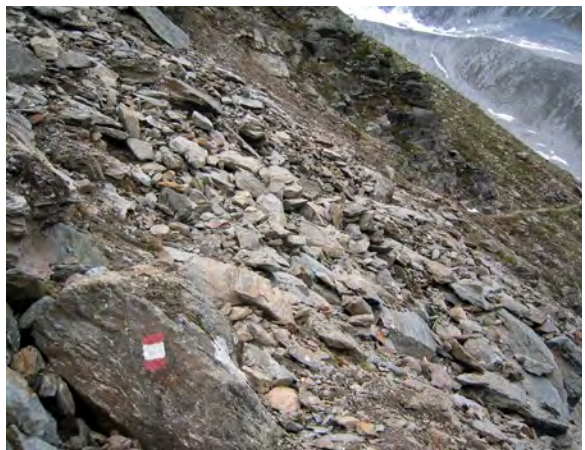
Fig. 9 Another portion of the same trail (represented in Fig. 6) partially buried under a deposit of debris and blocks. This is an example of a typical situation occurring at high altitudes at the beginning of the summer season. Due to the frequency of these instability phenomena, annual maintenance is required and, sometimes, new works after heavy rainstorms. This kind of hazard, if evidenced on geotourist maps, allows walkers to frequent trails with more safety. Moreover, public managers can use the same information to decide on modifications of the itinerary, temporary interruptions or in taking other decisions.
