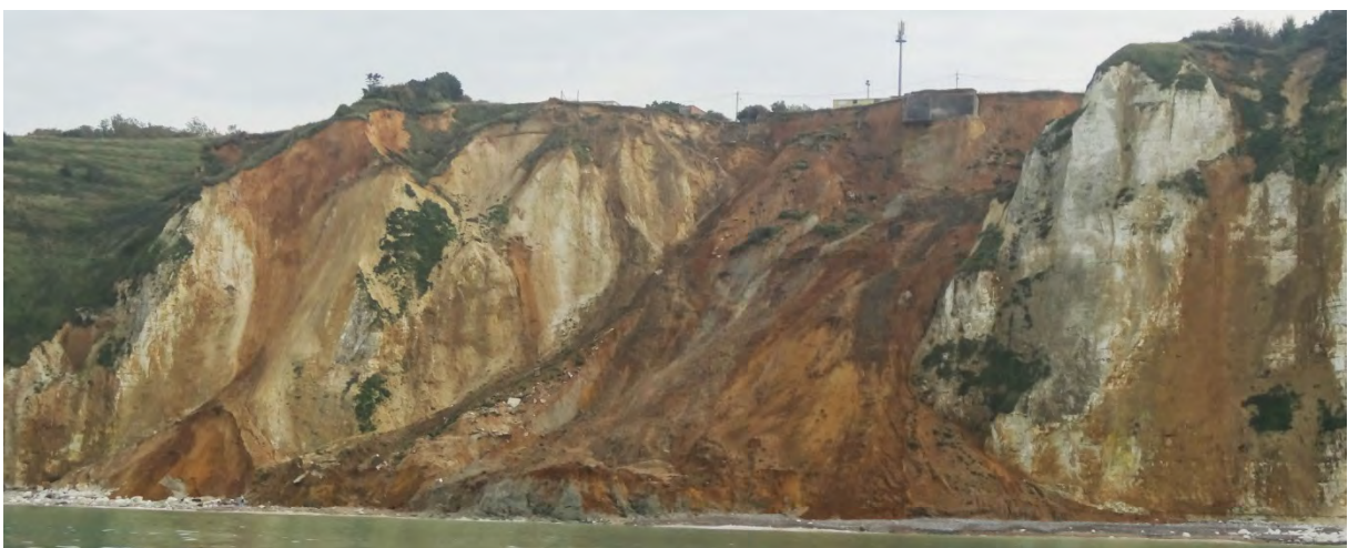
Figure 3.17: Picture of the Dieppe landslide in September 2013; the mass movement destroyed several constructions close to the shoreline after its activation in December 2012.
