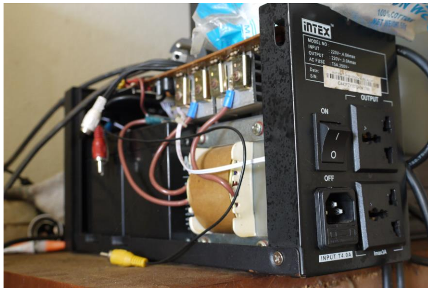
Figure 3 : Small UPS (Uninterruptible Power Supplies) are frequently used to provide emergency power to a load when the http://en.wikipedia.org/wiki/Mains_electricity fails. Many of them are damaged by electrical surges like the one on the picture above.
