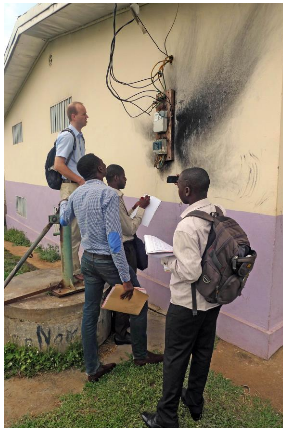
Figure 2 : Inappropriate electrical wirings or unbalanced/overcharges phases are causing many fire in electrical installation like on the picture taken in one of the audited hospitals.
