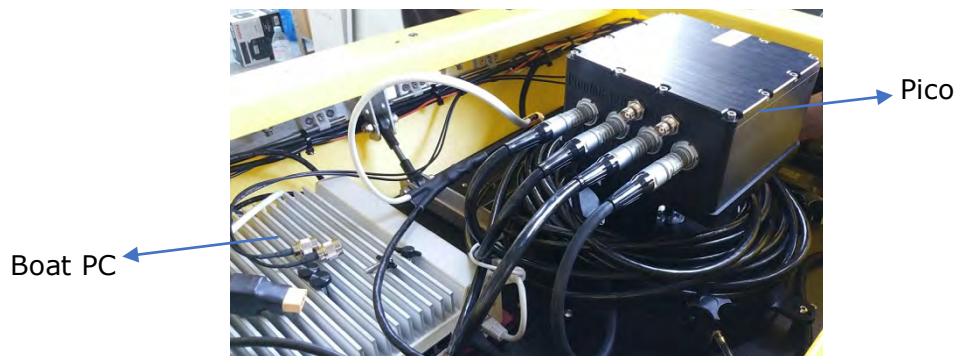
Figure 9: boat PC installed near the Pico
