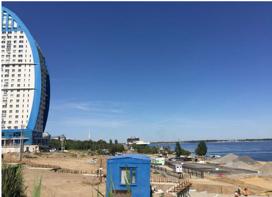
Figure 18: Construction of the new prodolnaya , or parallel road, along the banks of the Volga River about 5km south of Volgograd's World Cup stadium, next to a pair of elite apartment buildings. Source: author.
