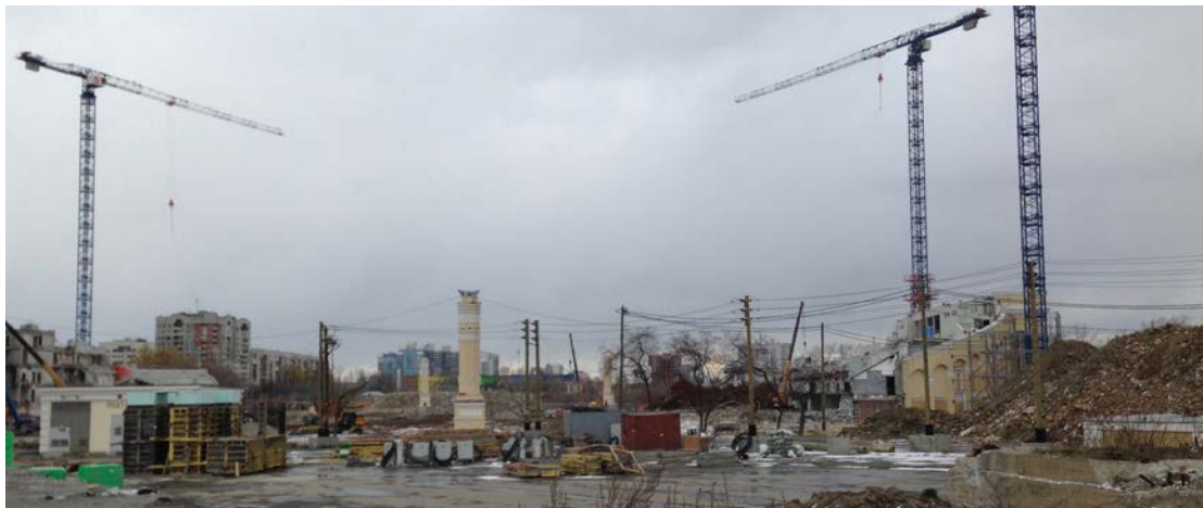
Figure 34: Remnants of the newly reconstructed and then demolished Central Stadium in 2015. Only the protected façade remained, along with a pair of columns. Everything else would be rebuilt from scratch, even though the previous reconstruction had just been completed in 2011. Source: author.
