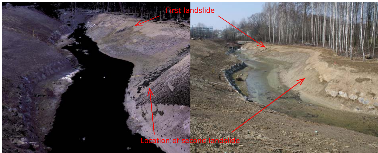
Figure 1: Views of the Sorge River to the West (taken on March 16 th 2006). The point cloud of the laser scanner and the photograph show the area of the remedial works that were done in 2005. The scar of the first landslide is also shown.
