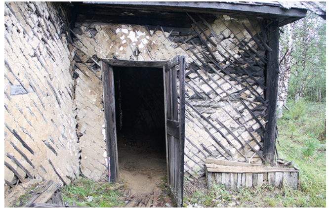
Figure 7. The entrance door to the eastern airlock of barracks B5. On the right, the insulation box. Remains of lime plaster are visible above the door (J. André).
