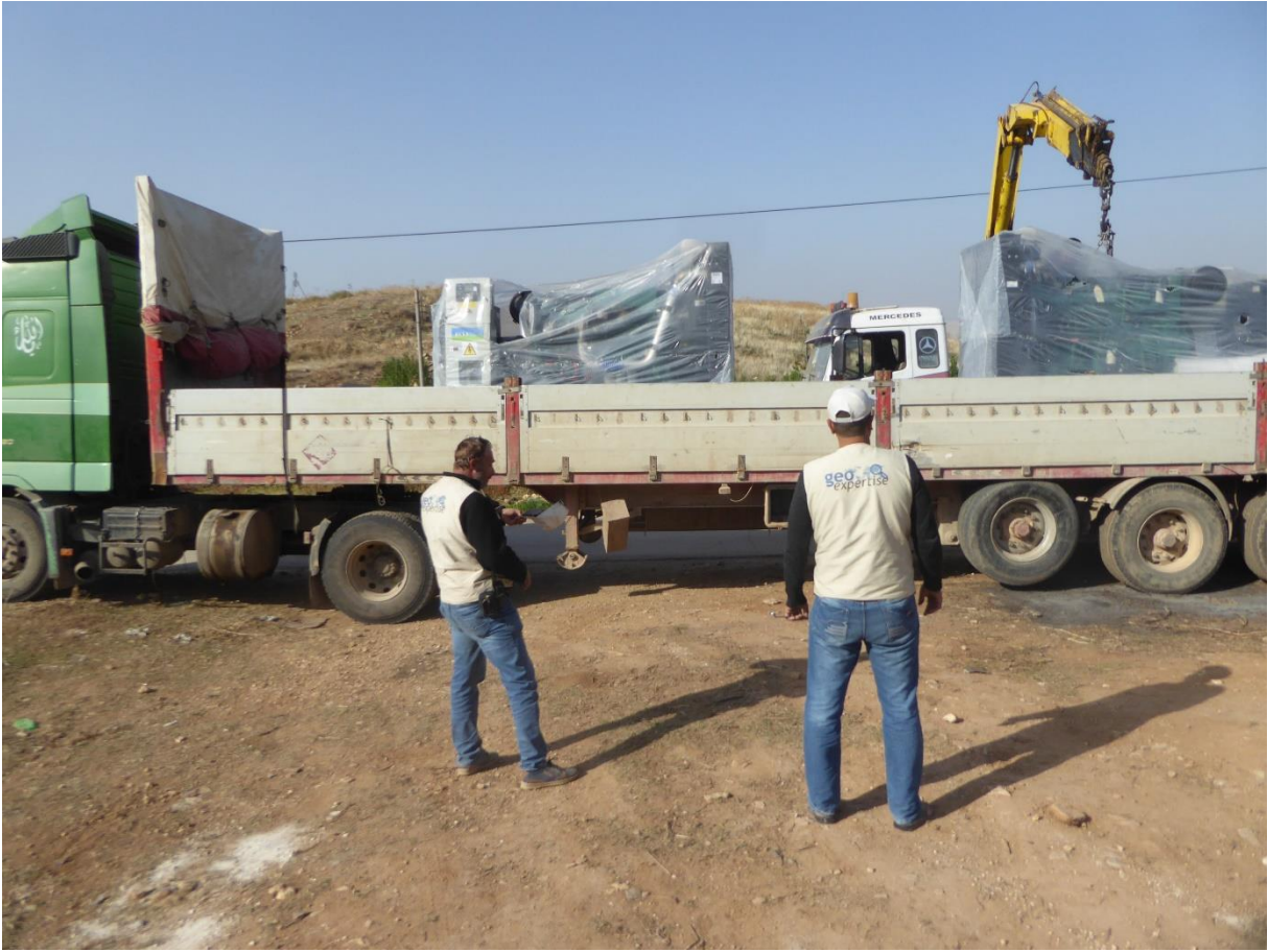
Figure 6.2. 15: Installation of two electric generators (Photo, Geo Expertise, February 2018)
