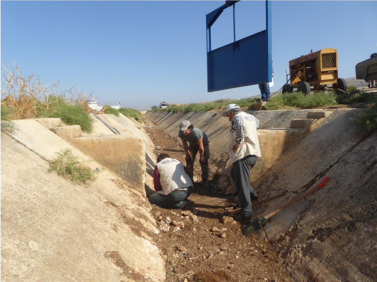
Figure 6.2. 12: Repair or replacement of the water distribution devices (Photo, Geo Expertise, August 2017)
