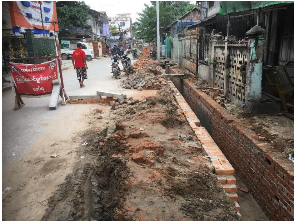
Figure 4. Brick drain in Pyi Gyi Tagon. Source: J.Sanchez
